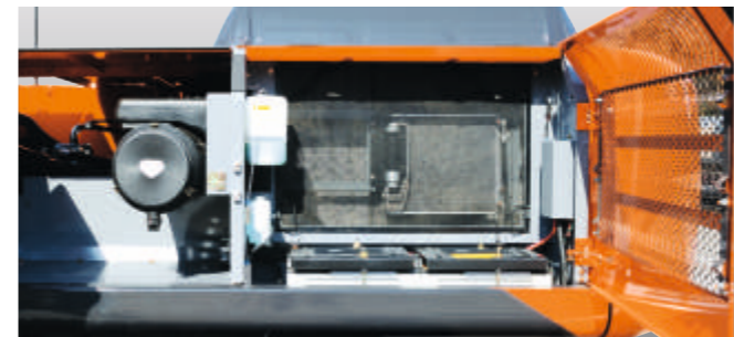
Utility space and radiators
